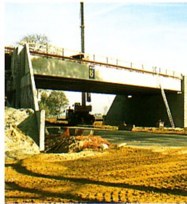
One of the several bridges that had to be built to link the farmland on both sides of the railway track.
