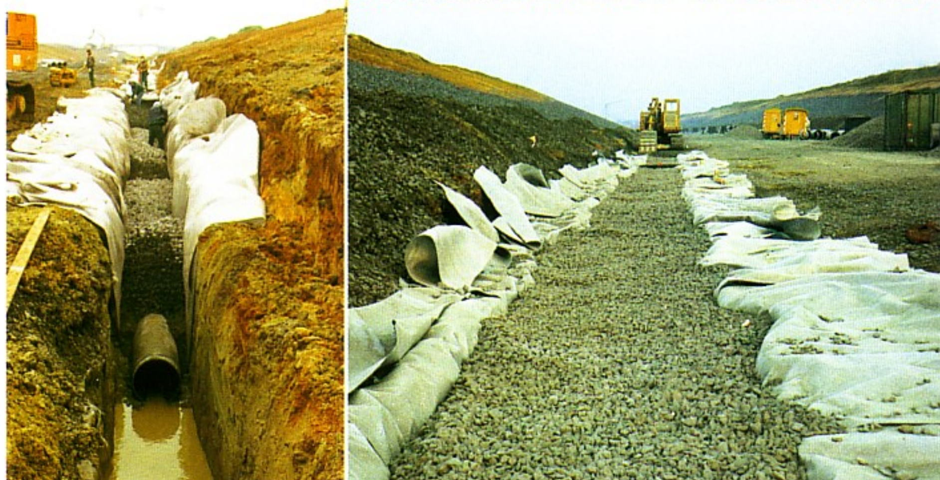
Typar® geotextile used in the trackside drainage helps to filter the ground-water.
