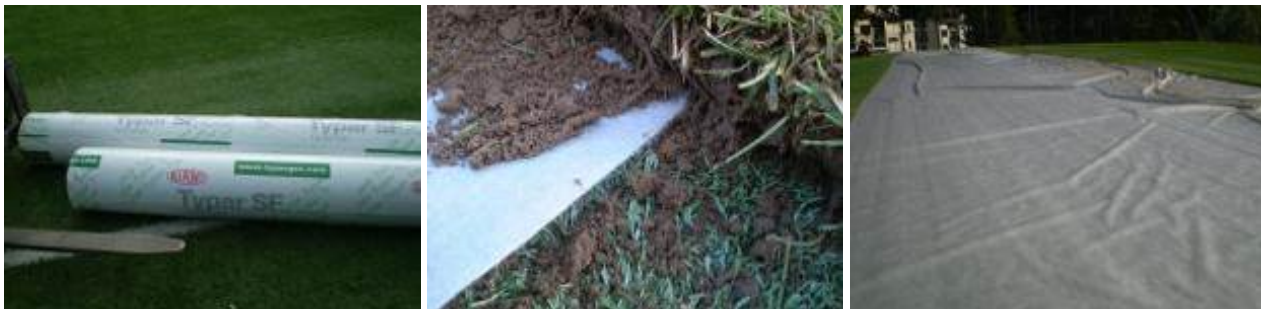
From left to right: rolls of DuPont™ Typar® ready to be installed; detail of the ground with DuPont™ Typar® geosynthetic applied; application of DuPont™ Typar® geosynthetic on the football field; photos by Bruno Marabotto, all rights reserved.
